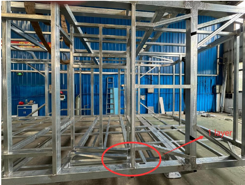
Other Factories--Disorganized framework, with minimal materials used, and sparse welding points
